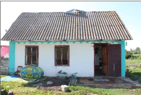
The tiny shed that is "home" for Tatiana and her family. The concrete footing is in place to add the entrance. Hopefully this will happen before winter.
